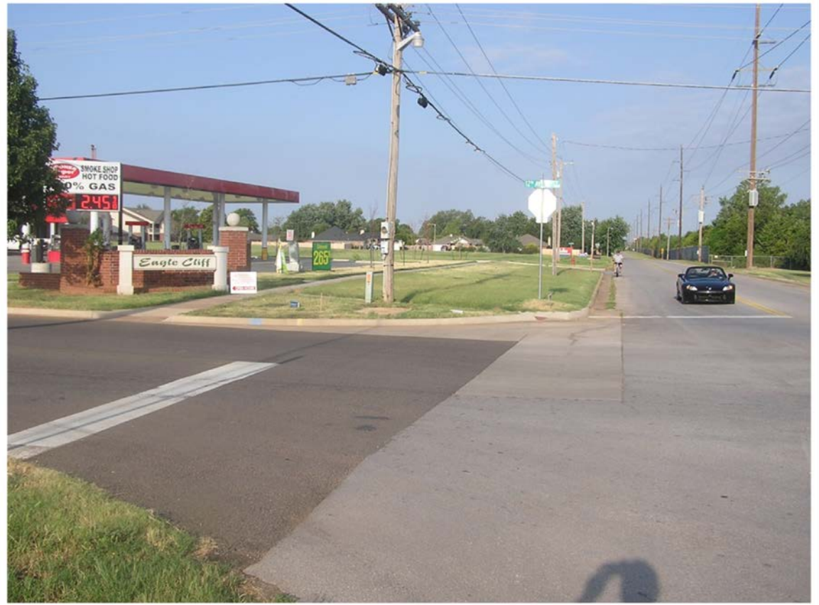
Four Lane Concrete Pavement on 12 th Ave 271' north and 490' south of Cedar Lane Ave
