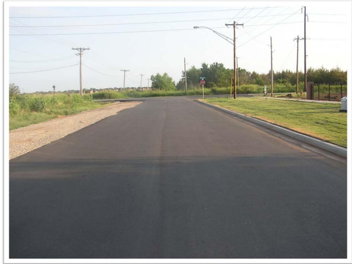
Four Lane Asphalt Pavement on 24 th Ave from Cedar Lane to 226' south
