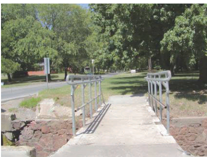
The Imhoff Creek footbridge at Boyd Street needs connection to the network of neighborhood sidewalks.
