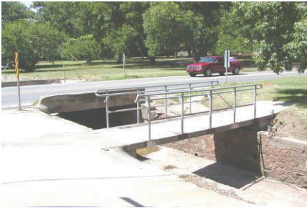
The street and pedestrian bridges over Imhoff Creek are in poor to sound condition. All modes of traffic circulation at this intersection need improvement.
